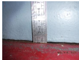
Panel to coaming clearance reduced
