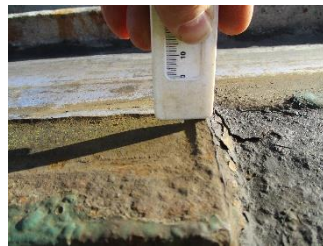
Bearing pad on coaming worn down
