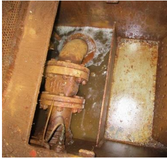
Backflow on bilge with strum box
