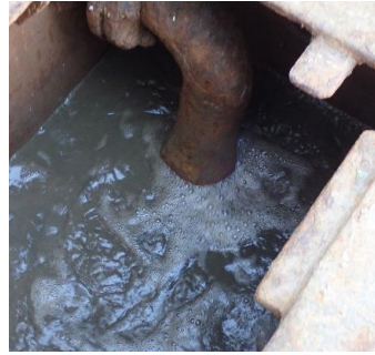
Backflow - no strum box fitted
