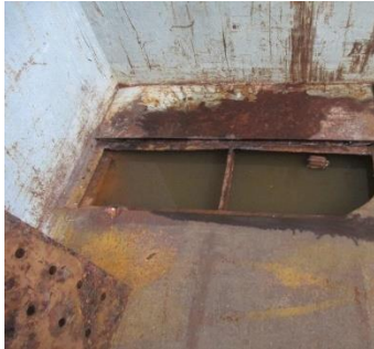
No suction - blocked pipe
