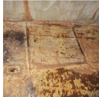
No suction - welded cover
