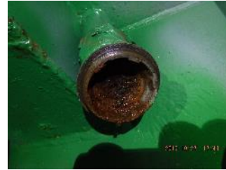
Drain valve, fire cap AND non-return system missing
