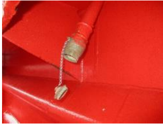
Drain valve with fire cap
