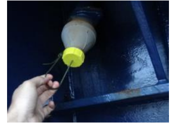
Drain valve, here with fire cap closed
