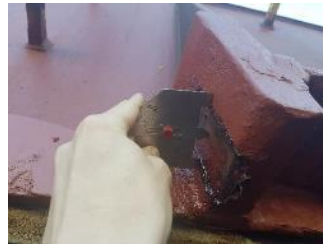
Weardown on hatch cover part of the structure
