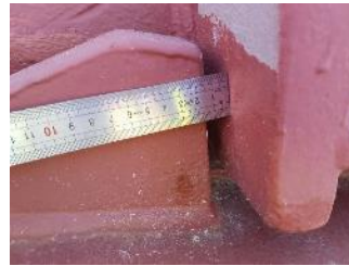
Measuring clearance on non-touching side to measure loss of steel on touching side
