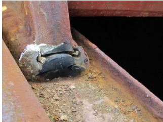
Perimeter rubber overcompressed
