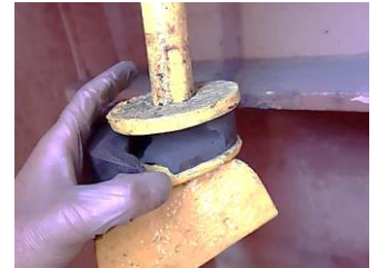
Cleat with cracked washer
