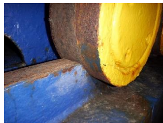
End wheel stuck on wheeltrack
